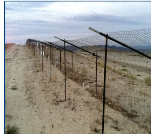
Example of a Horizontal Litter Trap Installed on a Temporary Litter Fence
